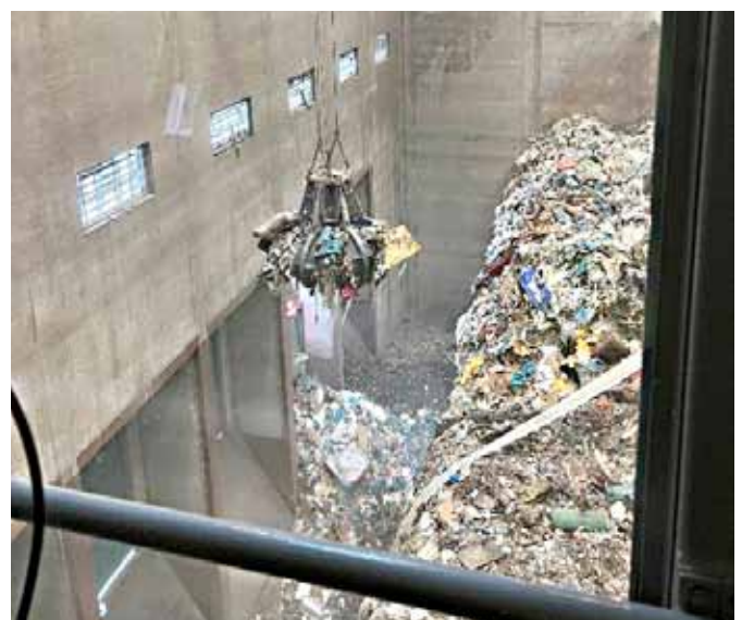
Blick in den Abfallbunker.
